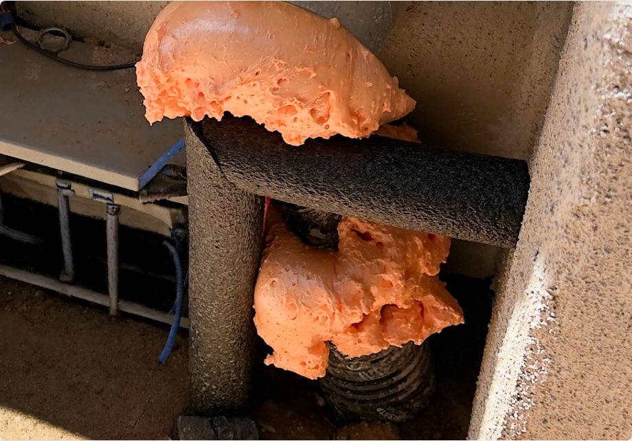
Class A Fire Rated Foam covered in foil for HVAC pipe gaps
